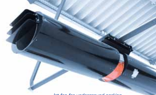
Jet fan for underground parking ventilation and smoke extraction
