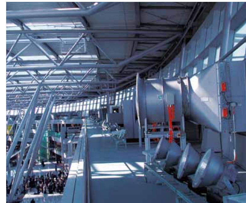
Exhaust fans at the Düsseldorf International Airport.
