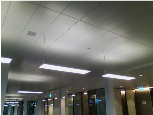
Metal chilled ceilings that cover
